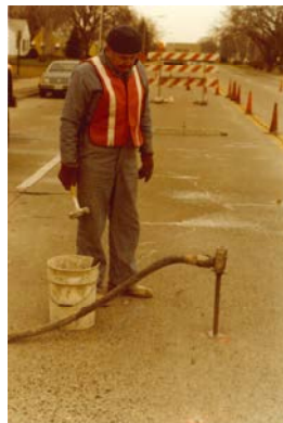
Concrete being poured under concrete slabs known as slab jacking Unknown location-c. 1970s
